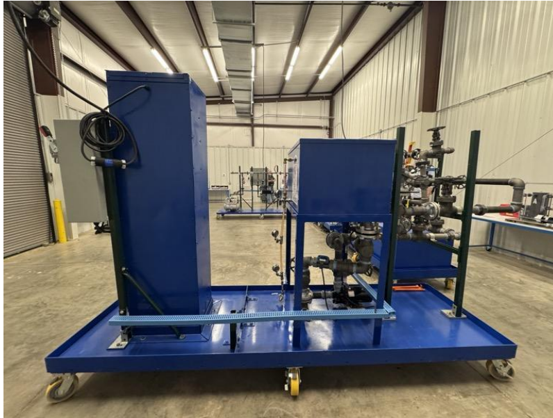
The reference: one of the real photographs of the test compressor skid.
